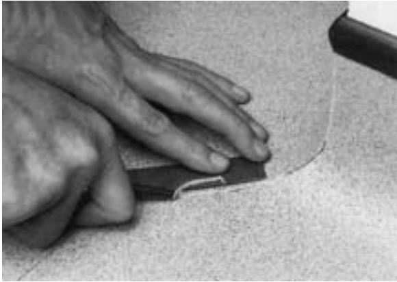
1. Groove the floor and bottom section. The top section of the mitre forms a natural 'Vee' and does not need grooving.
